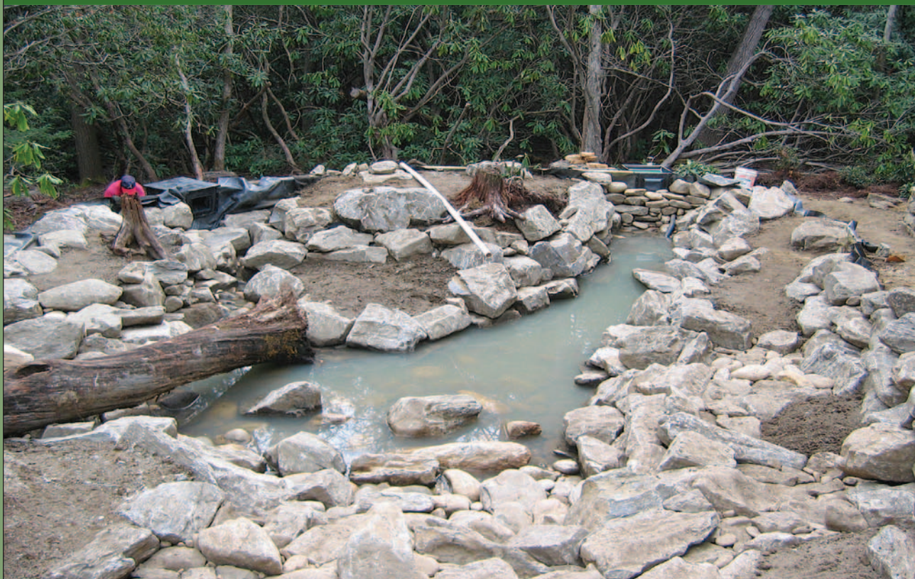
Rough in of two skimmers. Ponds of more than 8,000 gallons should use multiple skimmers.
