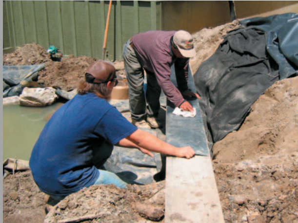
Use a 2"x12" board to make the cleaning and seaming process easier.
